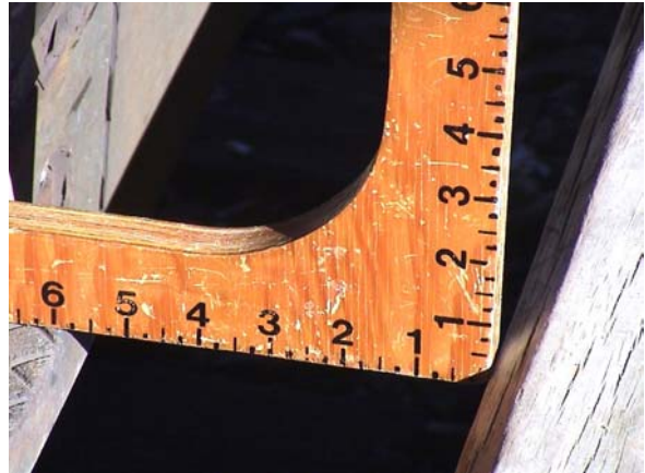
Tottenville subway station Showing a larger than acceptable gap
