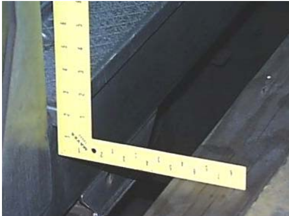
Simpson Street subway station Showing a larger than acceptable gap.
